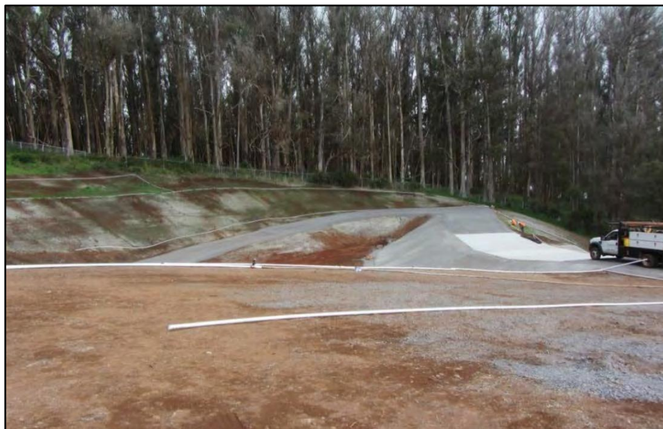
Olinda Sediment Drying Basin
