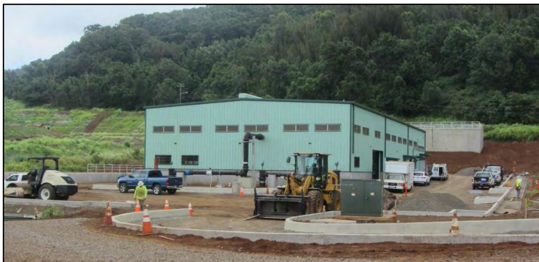
New lao Water Treatment Plant
